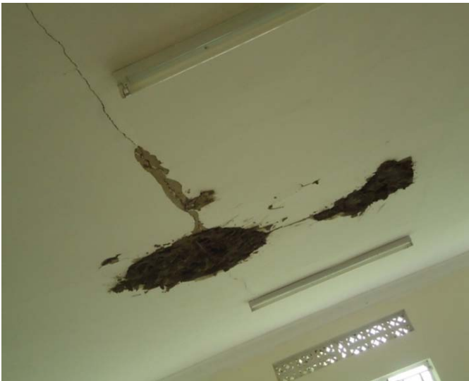
Ceiling before monitors' intervention
