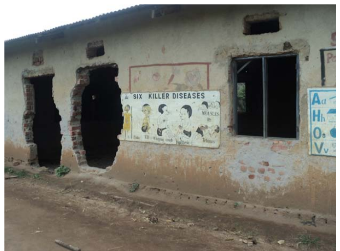
State of classroom blocks in a primary school in Harugale sub-county
