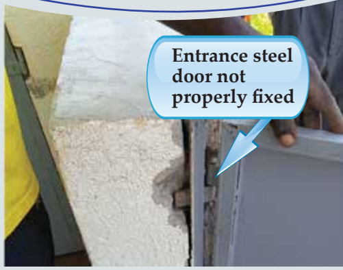
Defect on the entrance steel door
