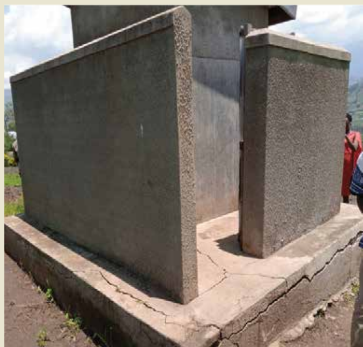
Cracks on the latrine before RAC intervention
