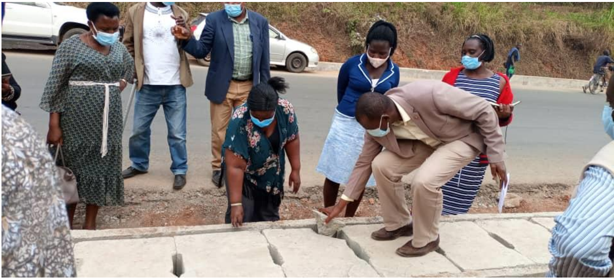
Figure 3: Fort Portal stakeholders during the joint monitoring visit of projects in Fort Portal (construction of water channels in Fort Portal)
